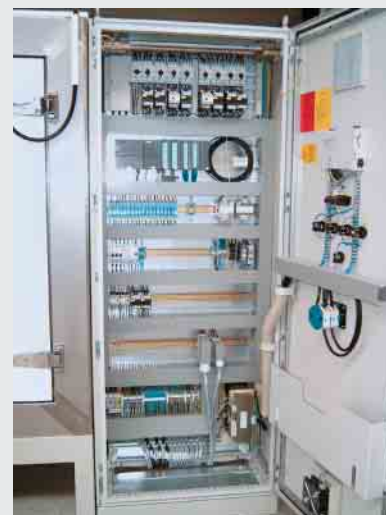
Switch cabinet with Siemens Simatic S7
